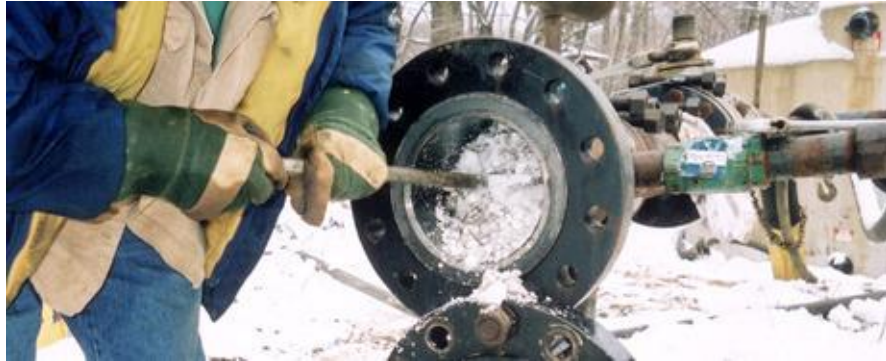
Figure 1.17: Gas hydrates removed from a pipeline [1.41]
