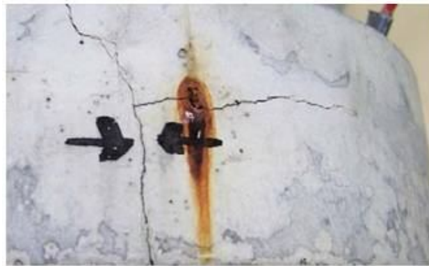
Fig.III-29. Creation of corrosion cracks from the intersection with transverse mechanical crack with reinforcement (duration 800 days) [22]
