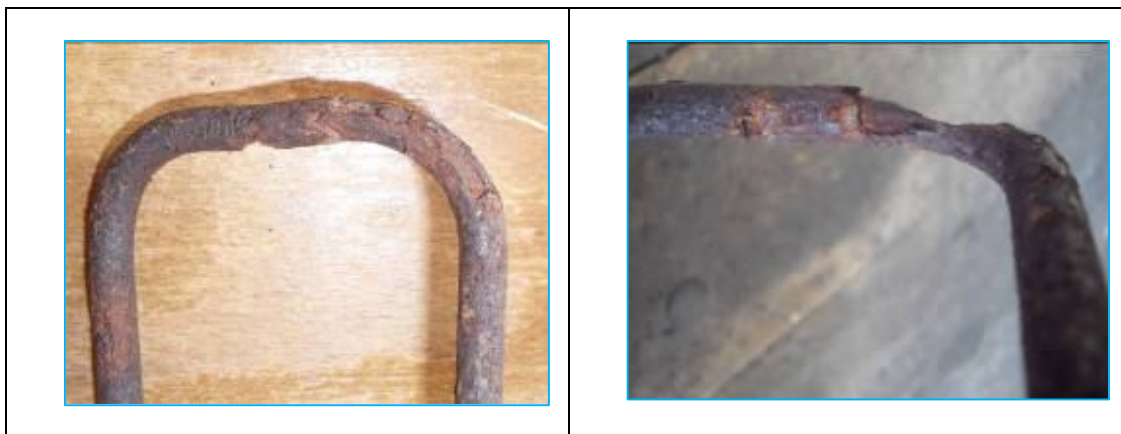
Figure 8. Real corrosion at upper part of stirrups
